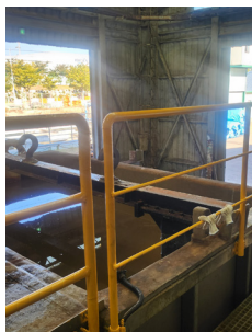
① Fall-Prevention Safety Fence
